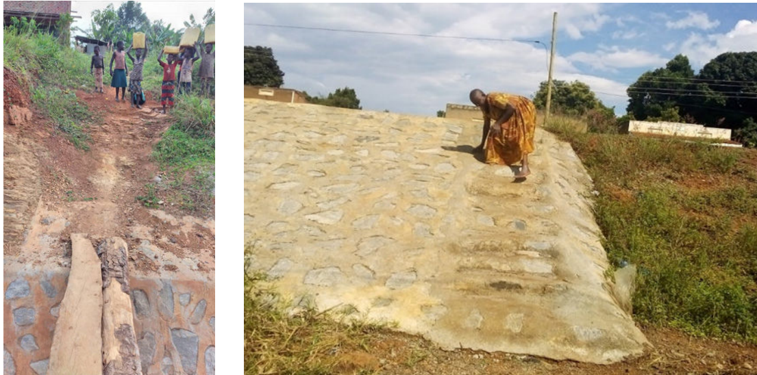
Figure 6: Pictures of inaccessible water along Buhimba-Kahumiro road, Kikuube district (Left) and lack of access to house due to poor construction at Buswekera, Hoima City (Right)
